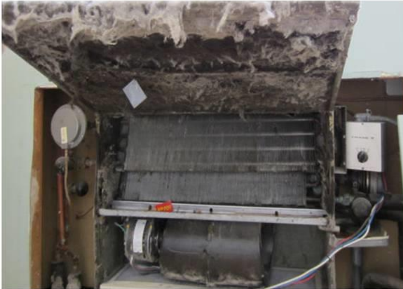
Photograph 4.4 Fan Coil Unit with Dirty Coils/Housing
